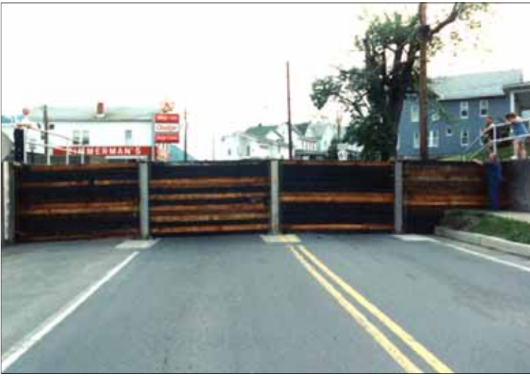
Wooden stoplog structure, Closure Structure No. 3, installed across East Market Street/Route 61.
