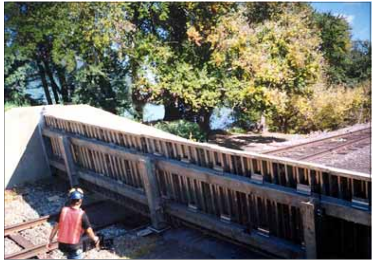
Aluminum "vertical" panel structure, Closure Structure No. 1, installed across the Canadian Pacific rail line at the North end of the city.
