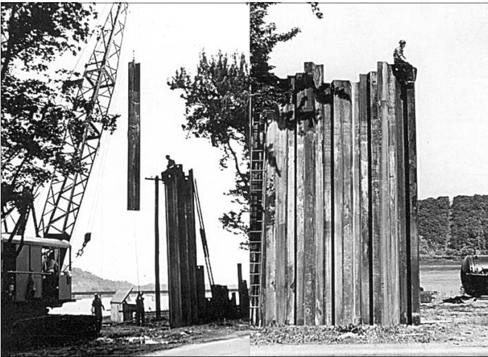
1947 Floodwall Construction - Steel sheet piling being driven into the soil to provide the foundation for the concrete floodwall.
