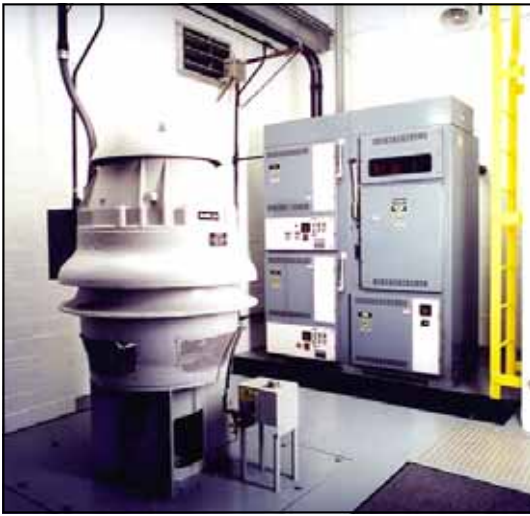
Hopper Alley pump station motor floor. One of the smaller river pumping stations.
