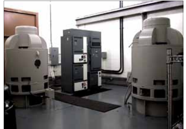
Spring Run pump station - Motor floor 2-350 hp motors with a pumping capacity of 47,500 gpm ea.
